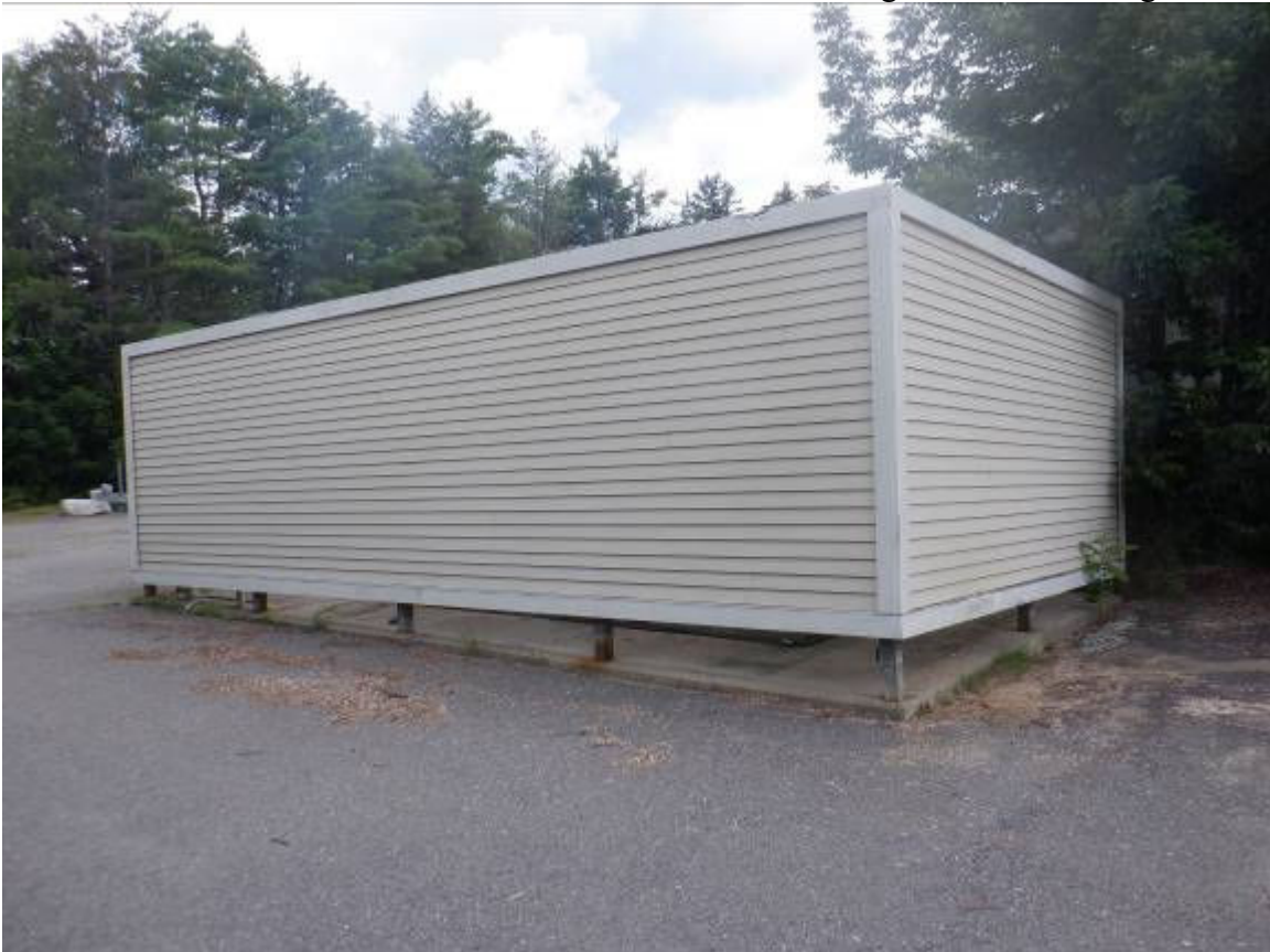
Wood frame structure around the A/C units for the original main building
