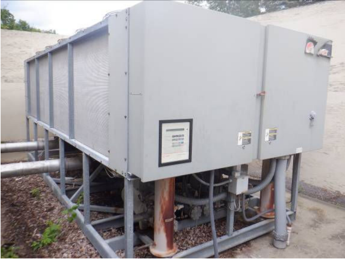
Main building A/C units
