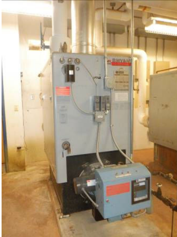
2 boilers – fuel oil fired
