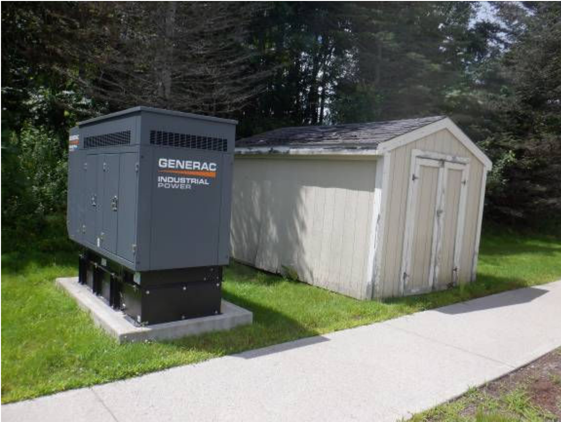
Generator and shed
