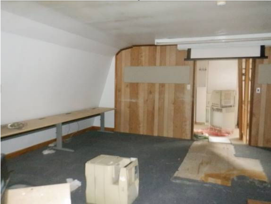
Second level – poor condition
