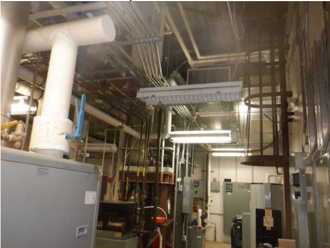
Utility room #1 – Room 110Y
