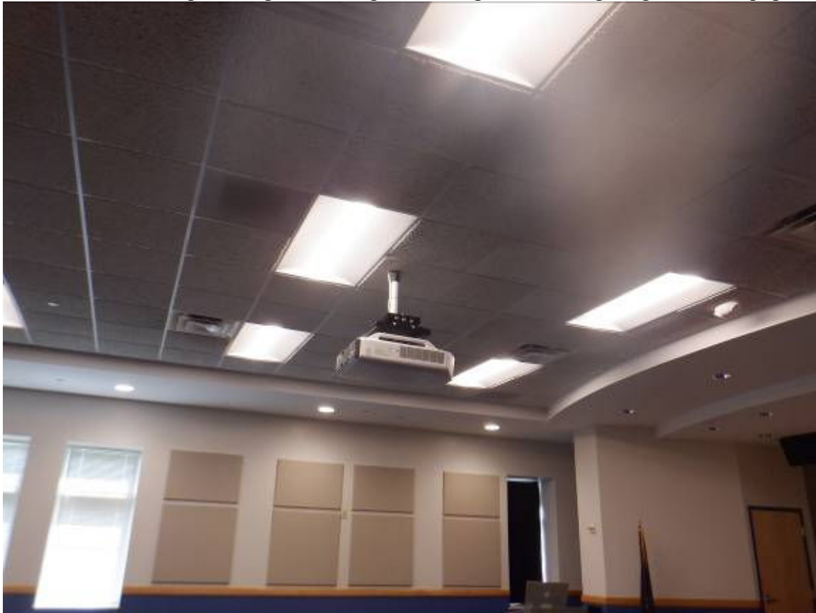
View of the reveal edge ceiling and ceiling HVAC registers, and lighting and AV equipment
