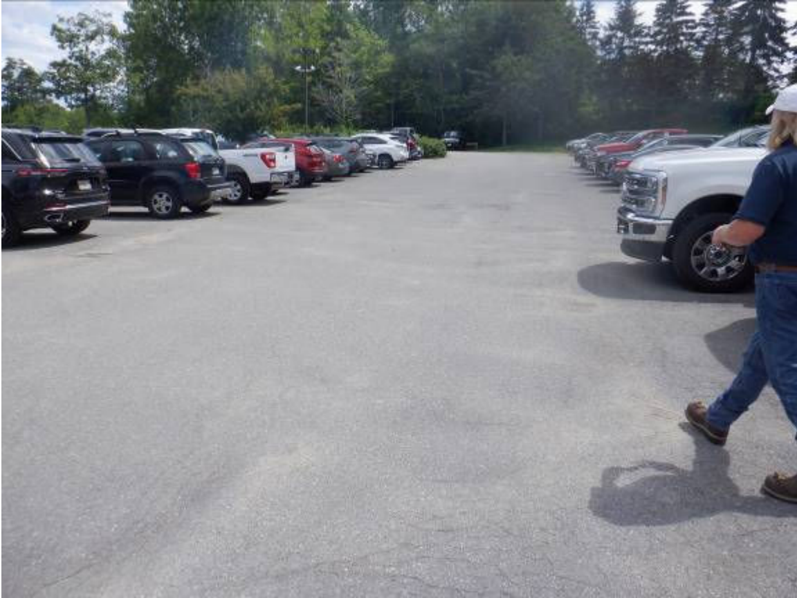
Parking area adjacent to the south wall; condition of paving
