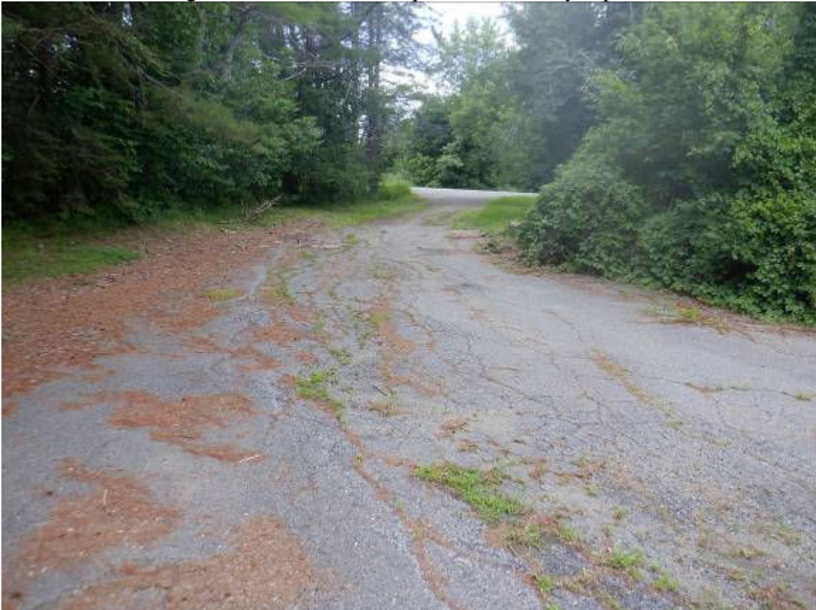
Parking area – condition of the pavement. Mostly depreciated.
