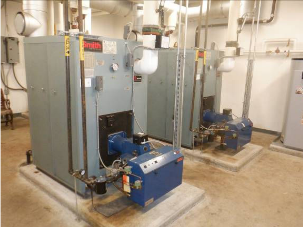
Boilers in Utility Room #2 (Room 126Y)
