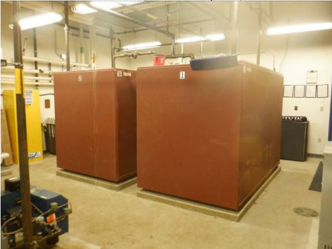
Fuel oil tanks (service both utility rooms)
