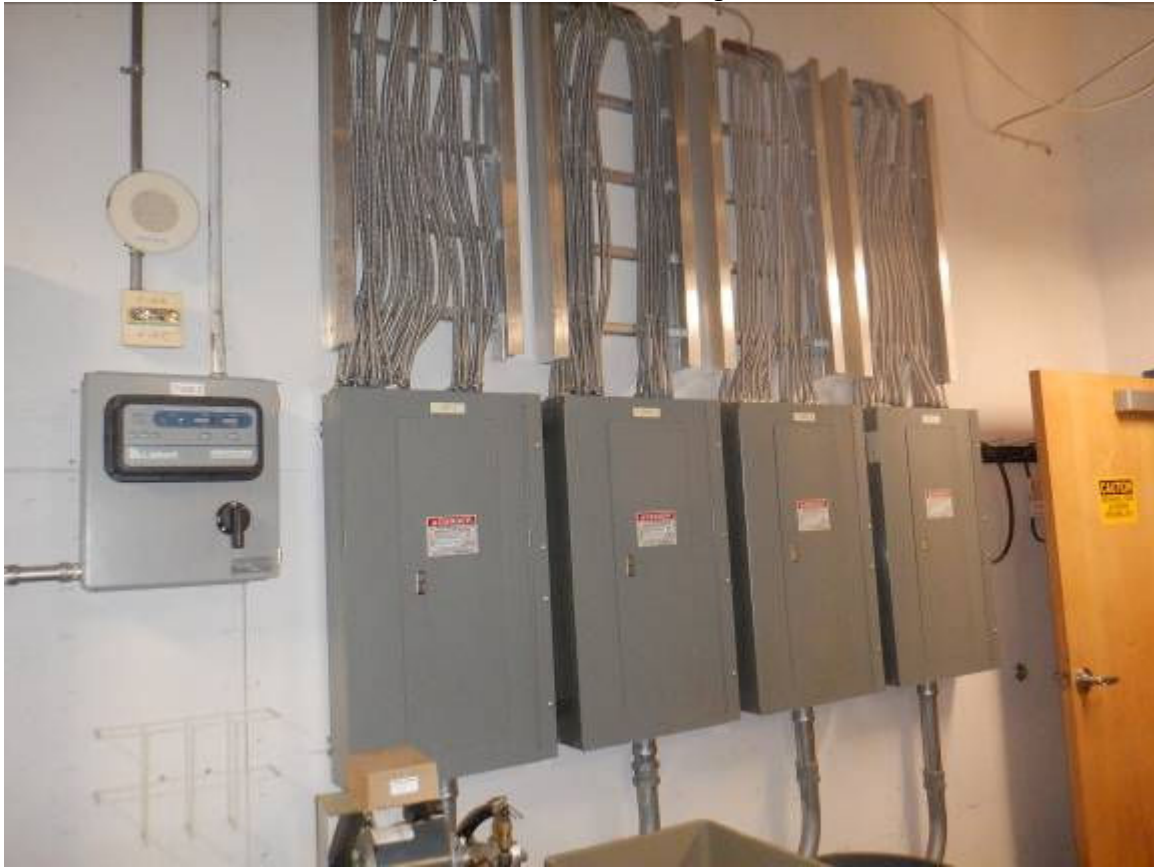
Utility room #1 and circuit panels
