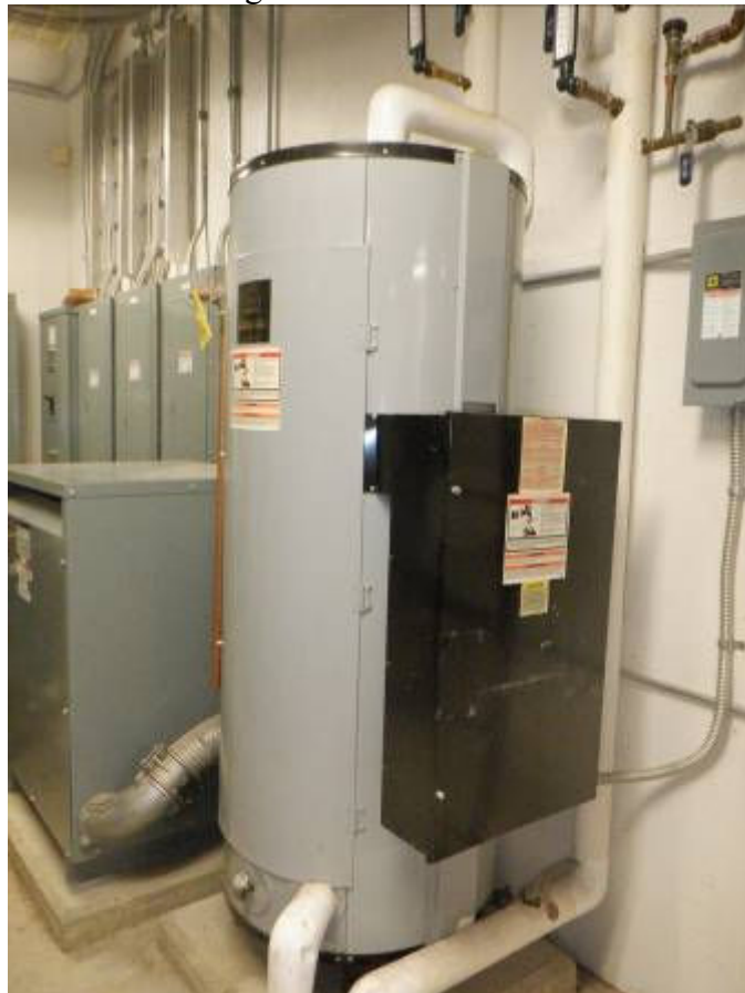
82-gallon hot water heater
