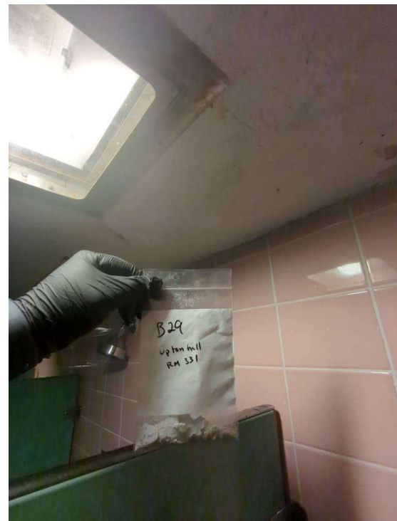
Upton Hall Wing Bathroom 331; Shower Ceiling Plaster
