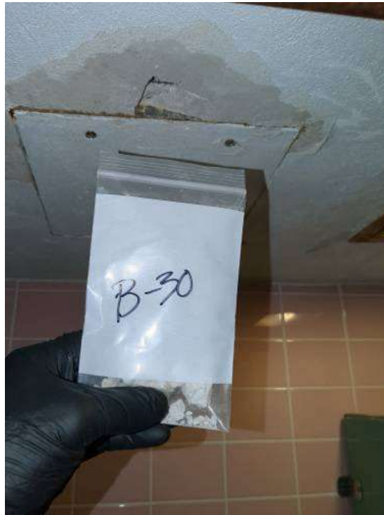
Upton Hall Wing Bathroom 331; Shower Ceiling Plaster
